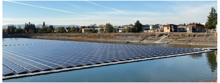
Floating solar array generates 73% of power for Windsor's Water Reclamation Facility
